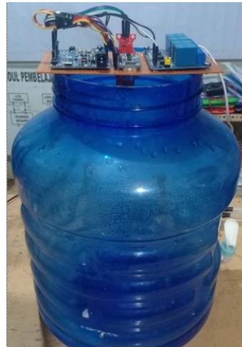
Fig. 7. Installation of a water level control system using an IoT application in a water reservoir
